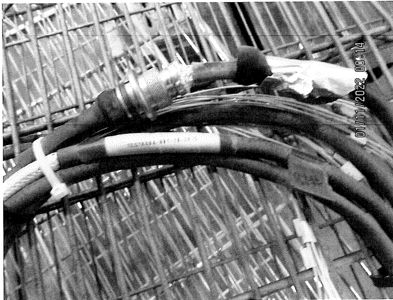
Photo 2 – File No. 0622-0012 Post-test photo Set 1
